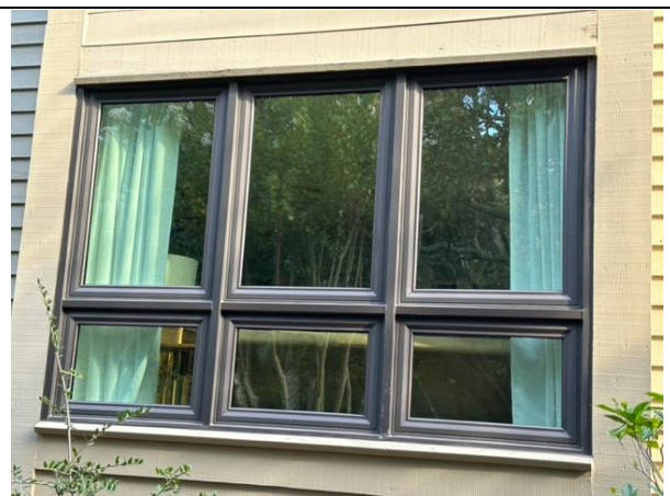
Figure 3a-2 Front (parking lot) Window
