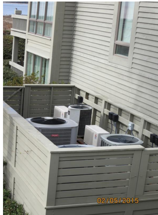
Figure 7b-2 HVAC Stand
