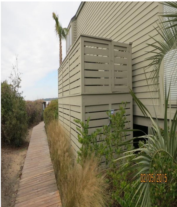
Figure 7b-1 HVAC Stand
