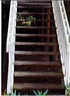
Figure 33 Original Stairs (no longer allowed)
