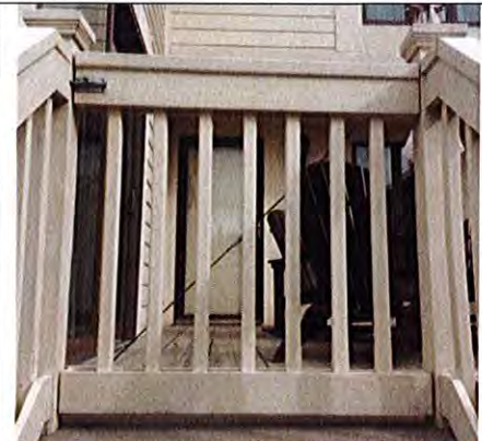
Figure 35 Approved gate at top of stairs
