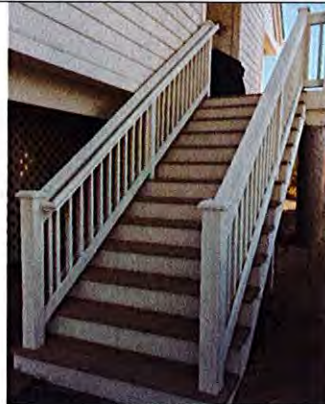
Figure 34 Required Stairs and Handrail (new style)
