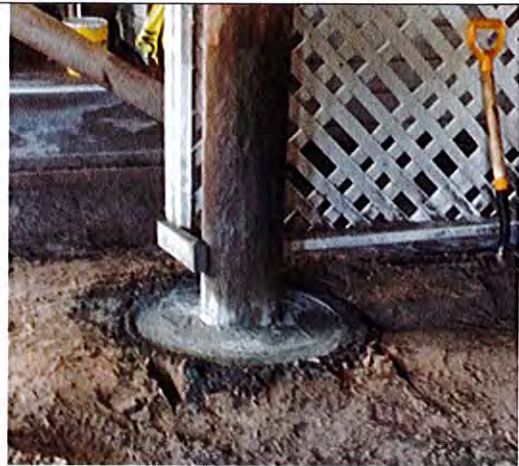
Figure 2 Piling encapsulation repair, another option
